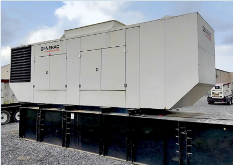
Used Generac 600 kW diesel generator model MB600.
