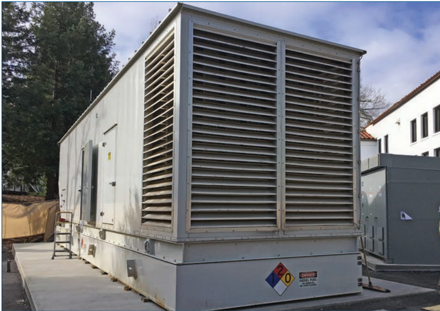
Caterpillar 2500 kW Standby Diesel Generator
