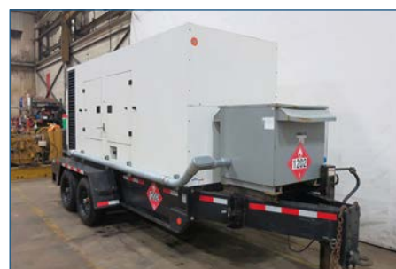
Doosan G325 Mobile Diesel Generator
