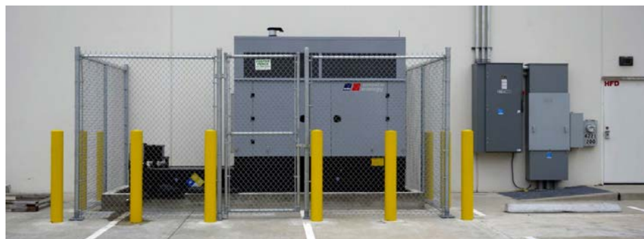
MTU Standby Diesel Generator and Asco ATS
