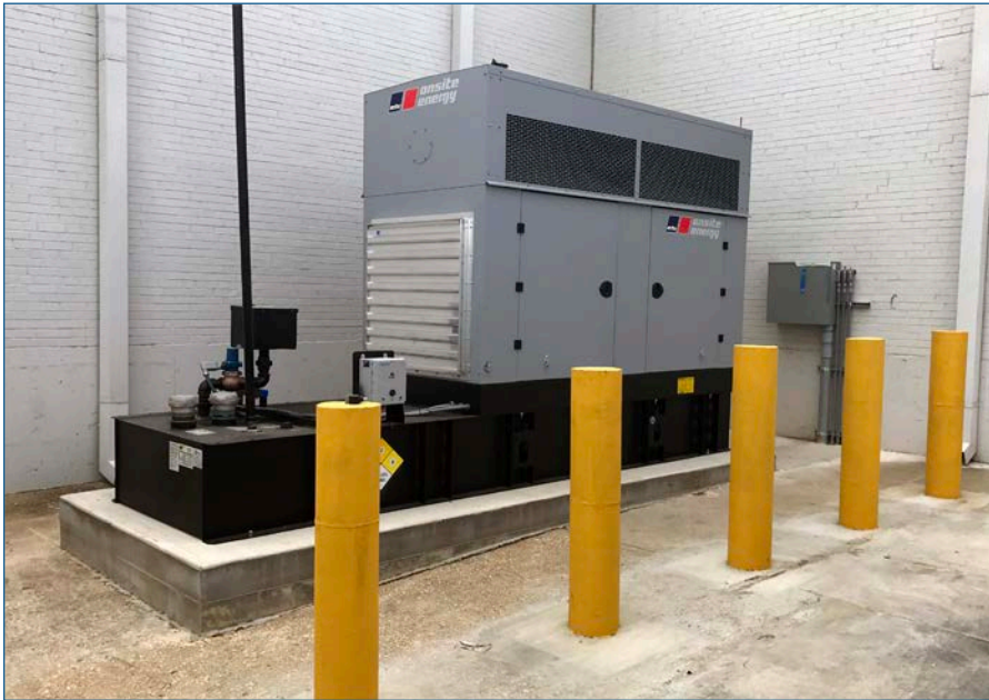
MTU Standby Diesel Generator
