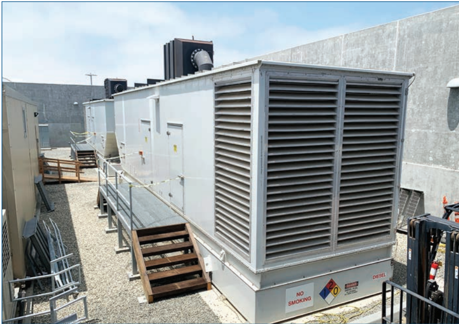
Caterpillar 2500 kW Diesel Generators at SoFi Stadium Inglewood, CA
