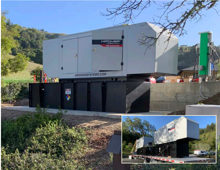
Global Power Supply Generator Turnkey Installation at Spirit Rock Meditation Center
