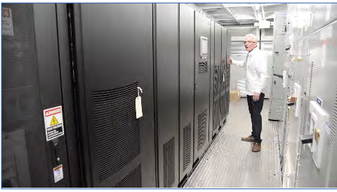
Interior UPS, Battery Cabinets and Switchgear
