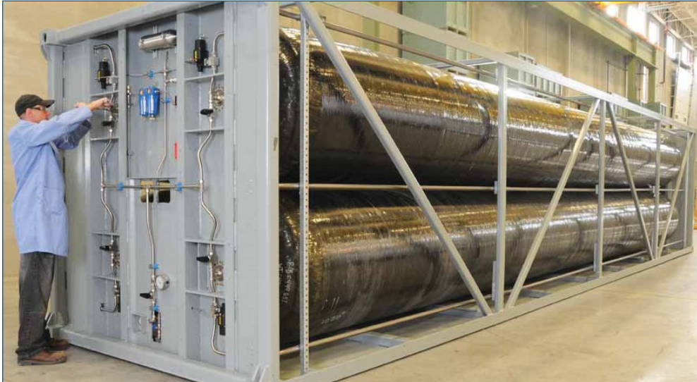
Micro containerized CAES systems for the delivery of stored energy volume for peak hours.
