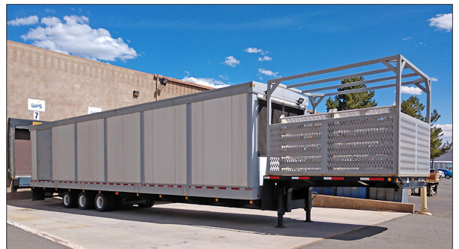
1200 kVA UPS Rental Trailer
