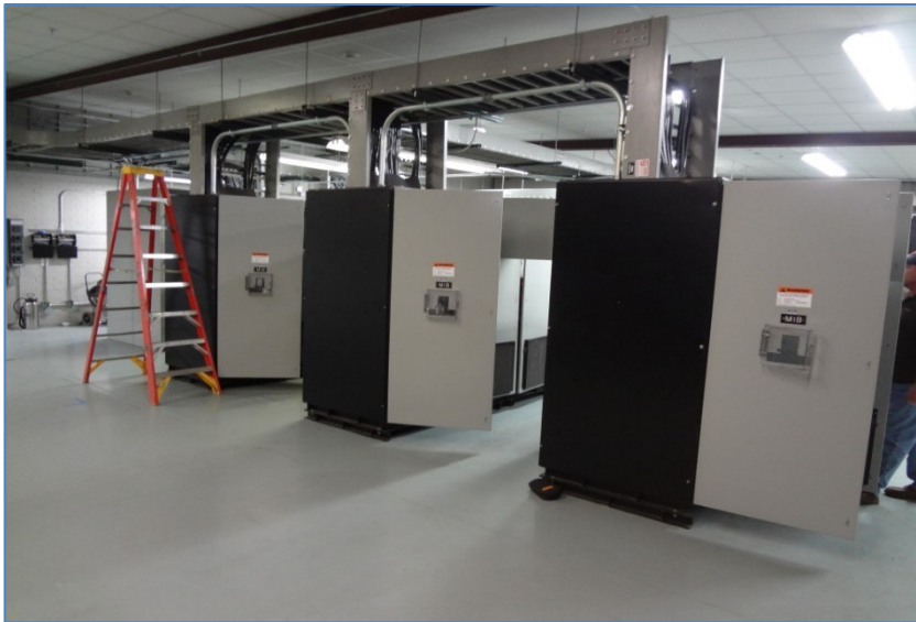
Existing UPS Systems to be replaced
