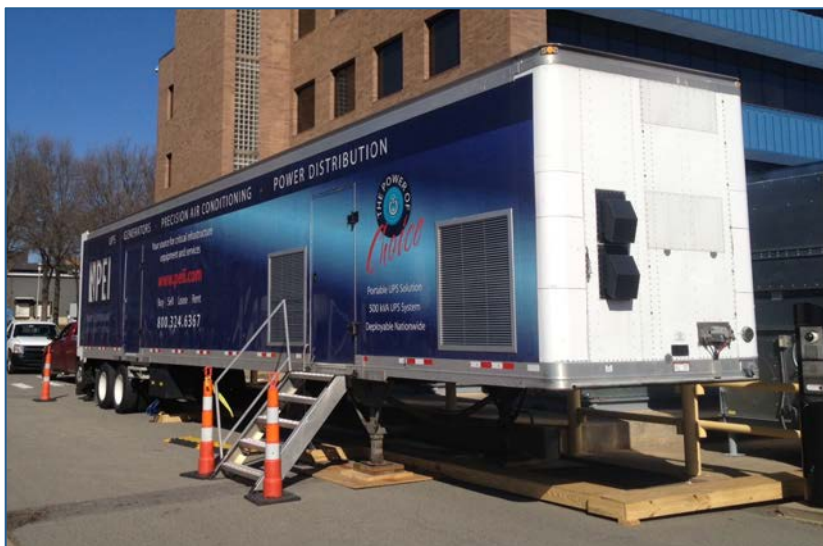
Self-Contained 1000kVA UPS System
