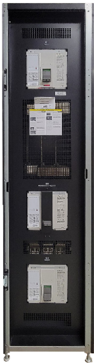
Maintenance bypass (door removed)
