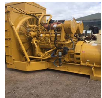
#6615 Caterpillar 1000 kW 3508B, Open Skid, Tier 0, 480V/60Hz
